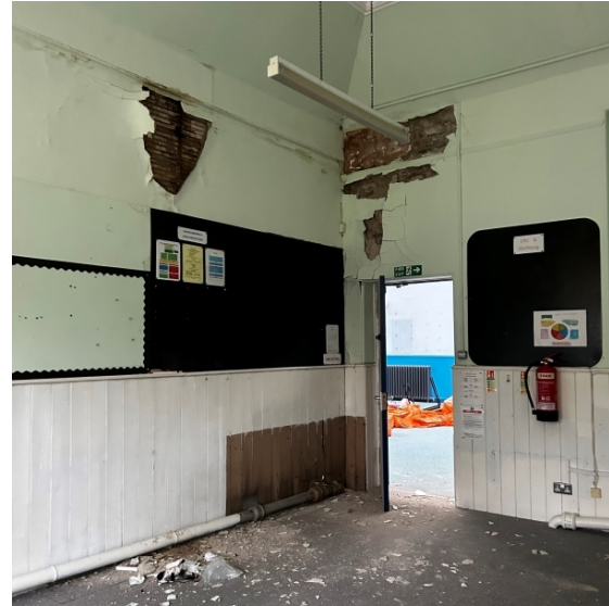
Classroom with crumbling lathe plaster walls
